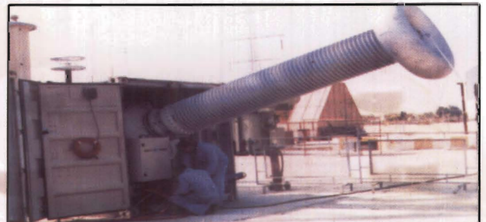
Fig (16) Mobile Test System 500 KV For on Site Measuring Partial Discharge
