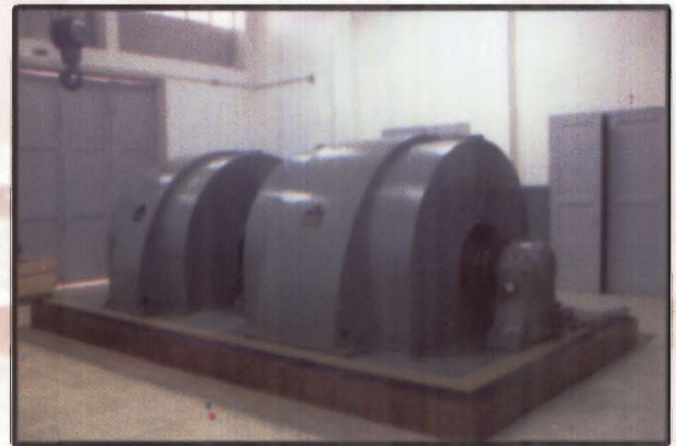
Fig (2) Motor Generator Set
