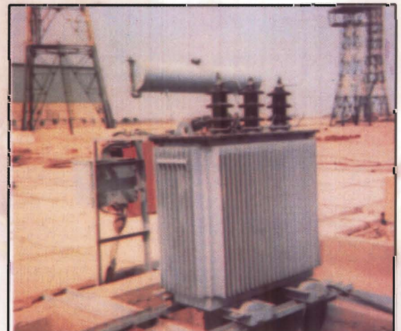
Fig (3) Test Transformer 20 KV - 150 c / s
