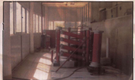
Fig (8) Impulse Testing Station 500 KV, 2.2 KJ
