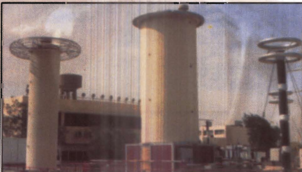
Fig (7) Impulse Testing Station 2400 KV, 180 KJ
