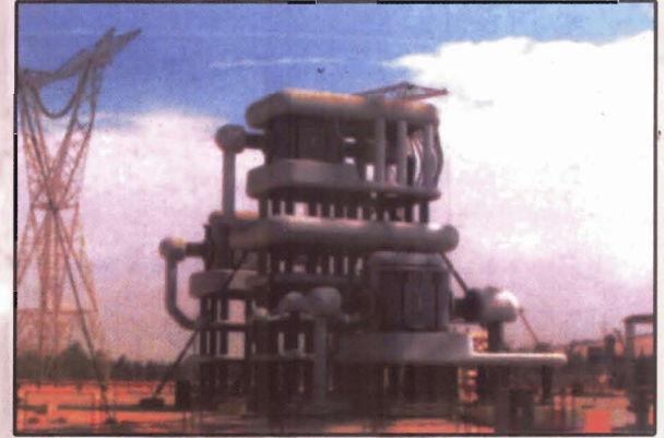
Fig (1) EHV Cascade Transformers
