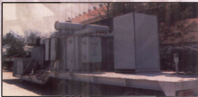
Fig (13) Mobile AC Testing Unit up to 100 KV
